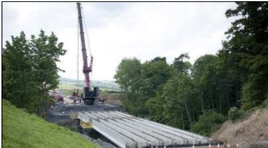
The pre-cast concrete beams positioned across the Langley Burn in Gee's Wood
