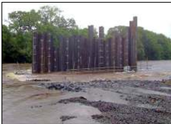
The June floods hamper progress on the construction of a cofferdam in the South Tyne, prior to work on the substructure of the viaduct across the river and the railway.
