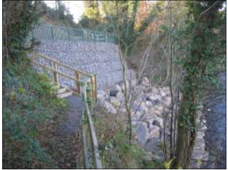
Looking west from what remains of the old path up towards the new platform. Several steps lead from the platform down to this level. The second landslide is just beyond this point.
